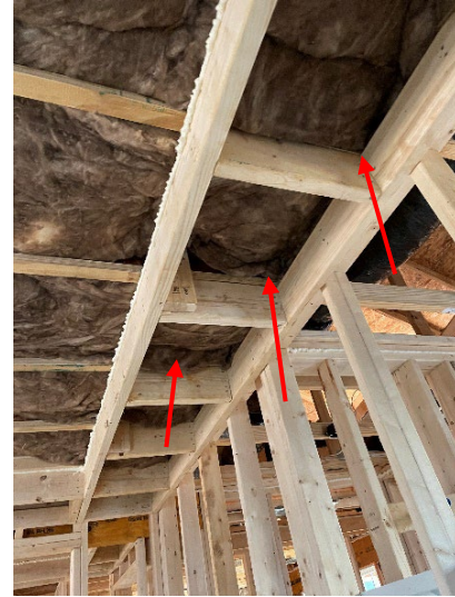
An improperly insulated dropped ceiling
