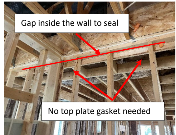
An example of an unsealed dropped ceiling
