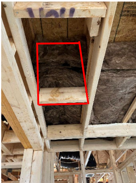
The red square highlights where an air barrier is missing in the dropped ceiling. The air barrier should extend from the subfloor to the bottom of the dropped ceiling where drywall will be hung.
