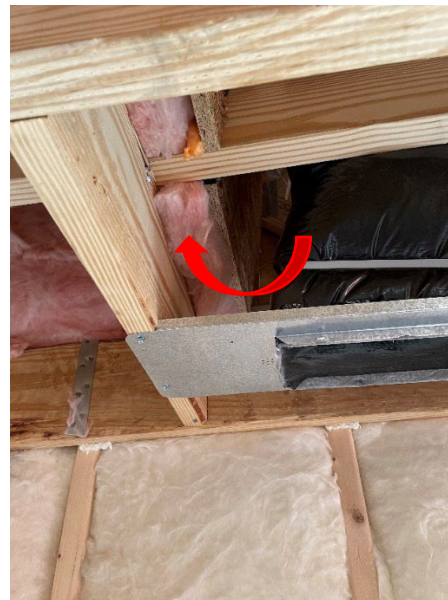
This example shows an air barrier was installed but does not extend to the drywall. The red arrow highlights the pathway for attic air to enter conditioned space.
