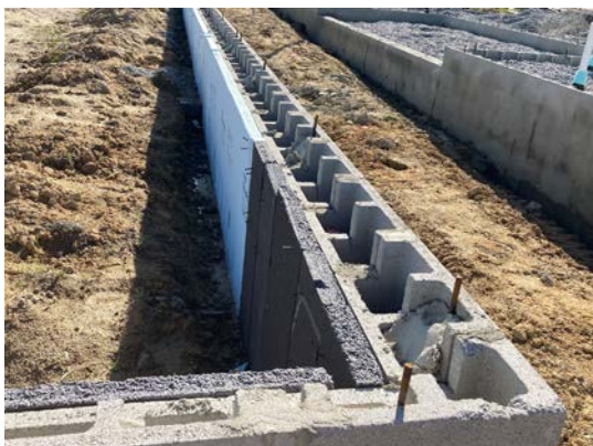
A stem wall missing insulation on the header block
