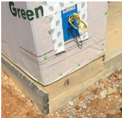
Misalignment of slab insulation on a garage foundation
