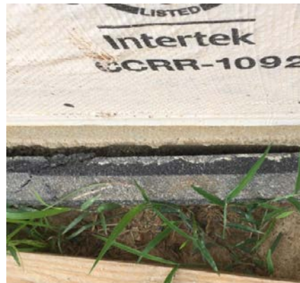
Slab insulation separated from the foundation
