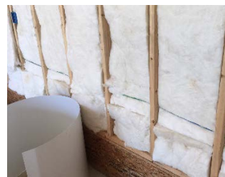
Insulation not split around termite obstructions
