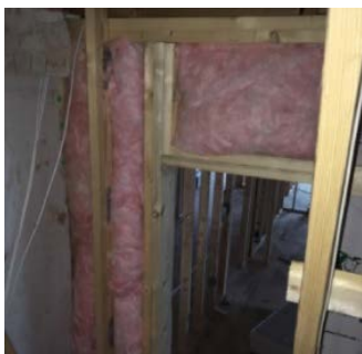
Kneewall missing an air barrier
