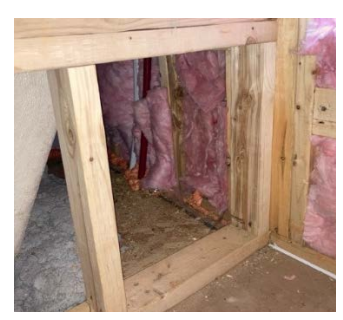
Tub missing an air barrier
