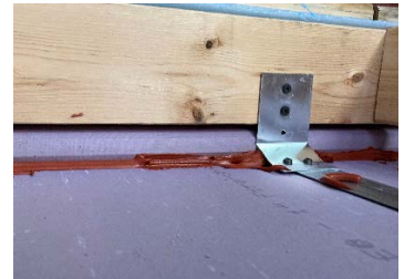
Core wall not sealed to top plates
