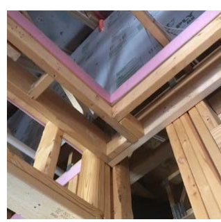
Dropped ceiling missing an air barrier at the top
