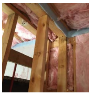
Double wall missing air barriers
