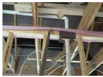
Sill seal installed on top plates with fasteners spaced more than 12"-16"
