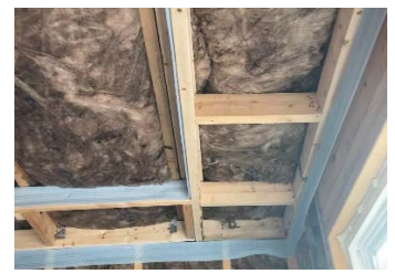
Insulation not installed to have substantial contact with drywall
