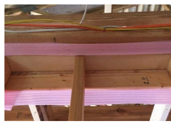
Dropped ceiling framing not sealed to top plates
