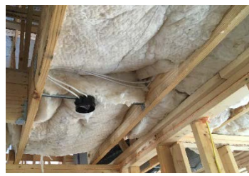
Ceiling insulation not split around obstructions or installed to have substantial contact with drywall
