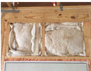
Insulation installed with compressions
