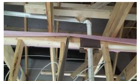
An example of incorrect staple spacing.
