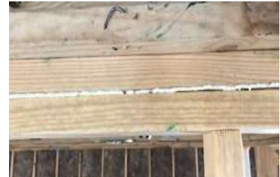
An example of incorrect bead size and location
