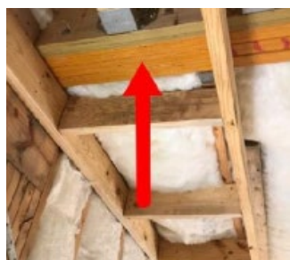
A knee wall rim joist in a dropped ceiling missing an air barrier.
