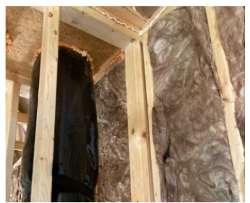
A chase on a wall backing unconditioned space missing a barrier.
