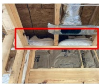
A garage floor rim joist missing blocking.
