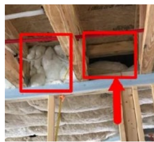
A kneewall rim joist missing blocking.
