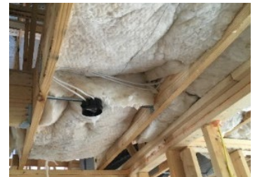
Ceiling insulation not making full contact with drywall.
