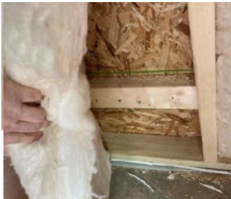
Insulation not split around wires and purlins.
