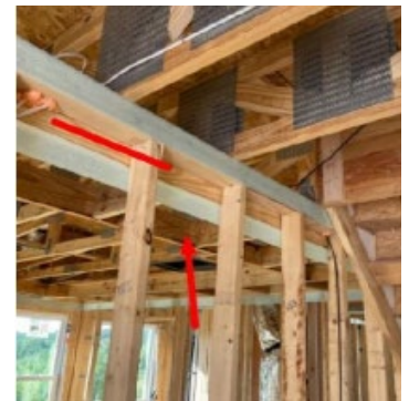
The framing of a dropped ceiling isn't sealed to top plates
