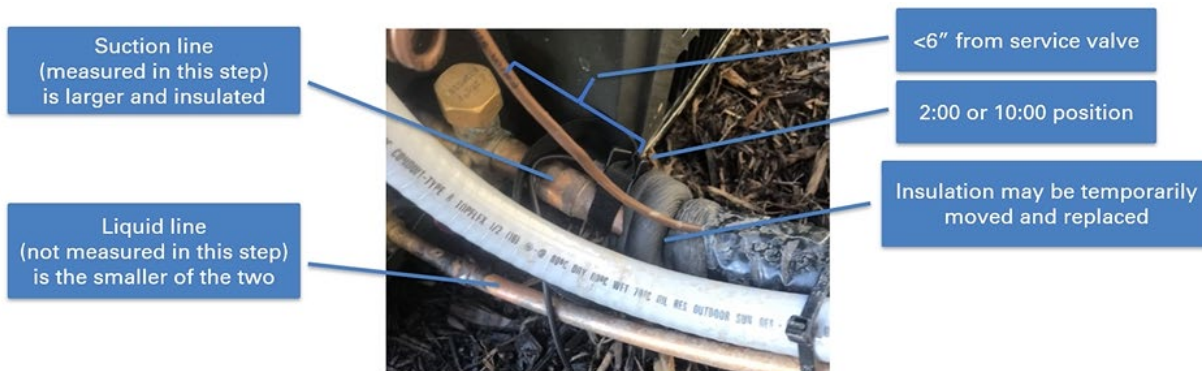
Image from RESNET shows the temperature test location and depicts the difference in the suction and liquid lines.
