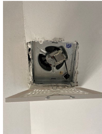
Bath fan exhaust is not completely caulked to the drywall.
