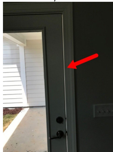
Rear door does not have weatherstripping.
