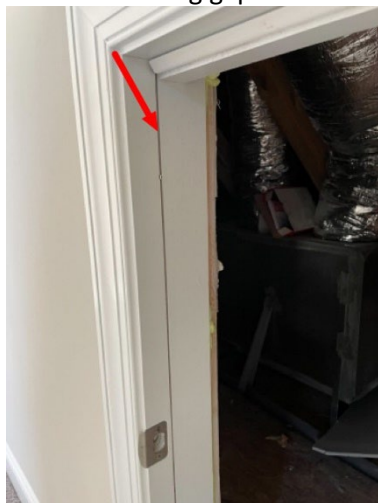
Attic scuttle door is missing weatherstripping on the sides.
