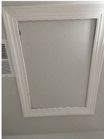
Attic scuttle is not aligned with the framing leaving gaps.
