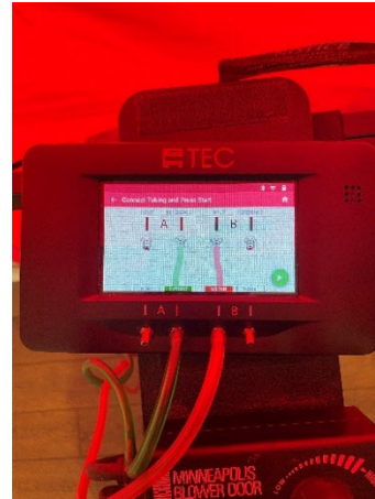
The DG1000 has a tubing assistant feature, this can be used to ensure hoses are connected correctly.
