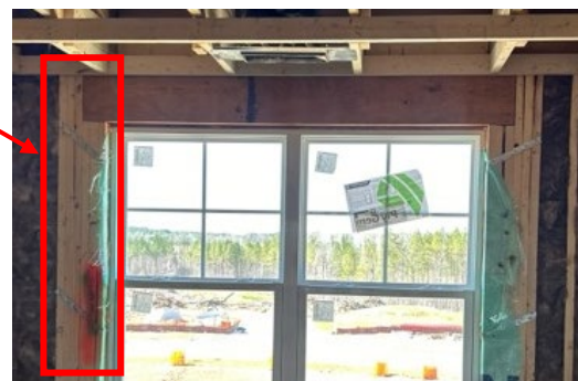
Two windows that are standard framed with three pairs of king and jack studs.
