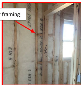
Ladder framing with thermal bridging preventing a fully insulated wall cavity
