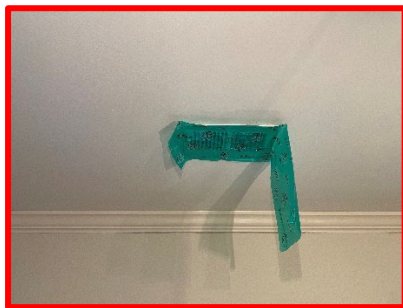
Tape only covers the supply, is not sealed to drywall.
