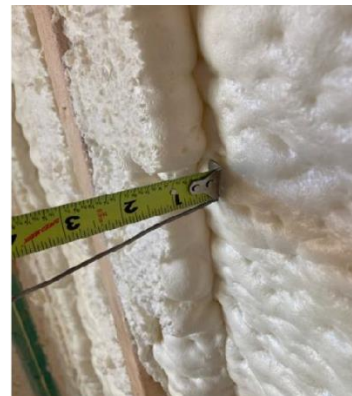
Figure 5: Example of insulation not filling a cavity completely.
