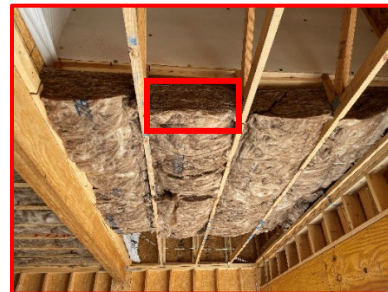
Kneewall rim joist above the garage is missing an air barrier.
