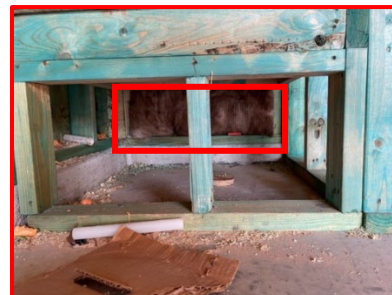
Chase under the water heater platform is missing an air barrier.
