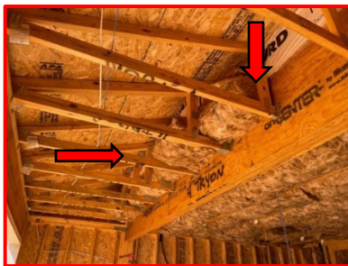
The floor above the garage juts out past the LVL beam and is missing an air barrier at the ends and side.
