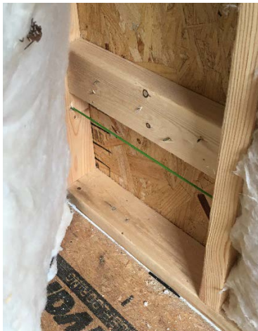
An example of termite systems and a 2x4 obstruction
