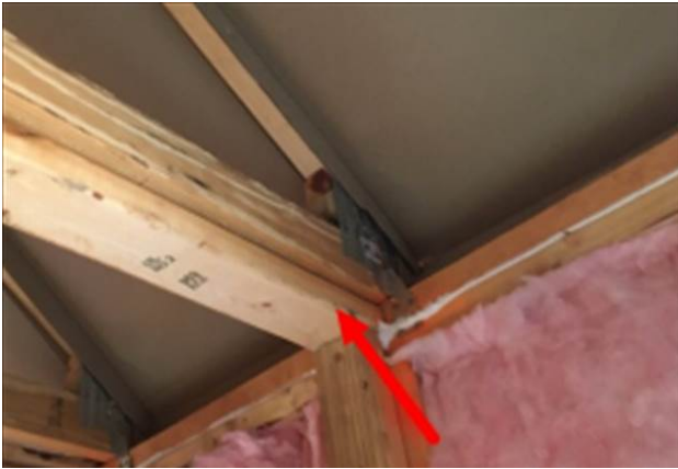
An example of top plate gasket missing on interior walls.
