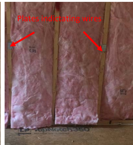
An example of batts not cut to fit wall cavities with plates showing wire locations
