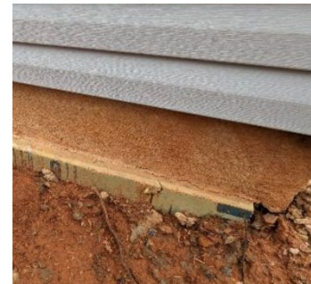
An example of a large termite gap
