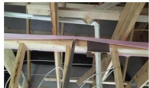
An example of incorrect staple spacing.
