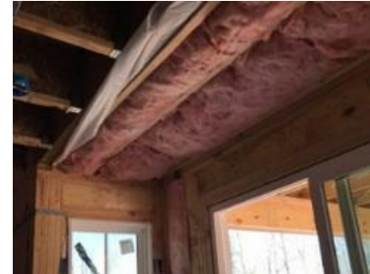
Top plate missing a gasket on the first floor
